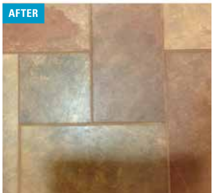
Before and after photos of grouted tile floor cleaned with green turf pad.
